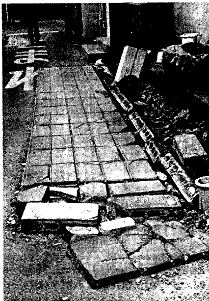
Fig. 10. Damage to unreinforced concrete block masonry garden walls.
